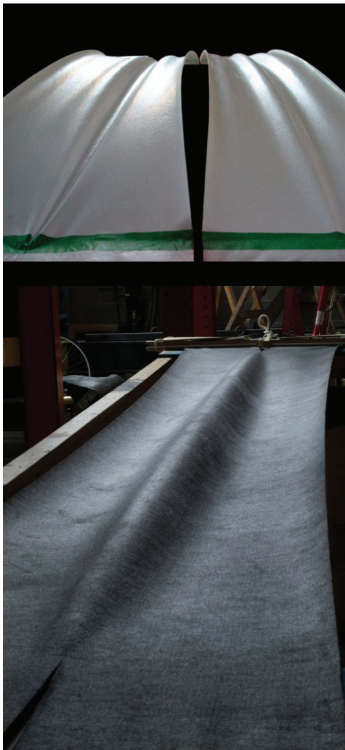
Figure 2. Plaster study models of fabric formwork vaults (top); Full-scale PE fabric formwork vault ready to receive application of concrete (bottom).
