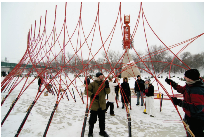
Figure 4. Fiberglass framing being installed on the frozen Assiniboine River in preparation for fabric formwork layer to be received.
